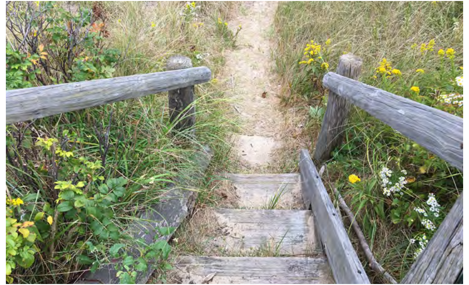
View of existing stairs which are in disrepair.
