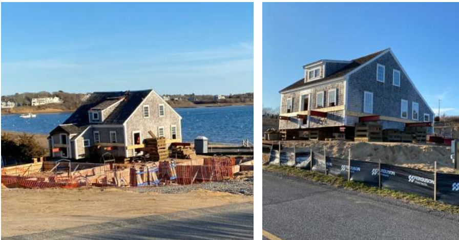
This historic house in Chatham was relocated on the same lot to preserve it while allowing room for new construction.
