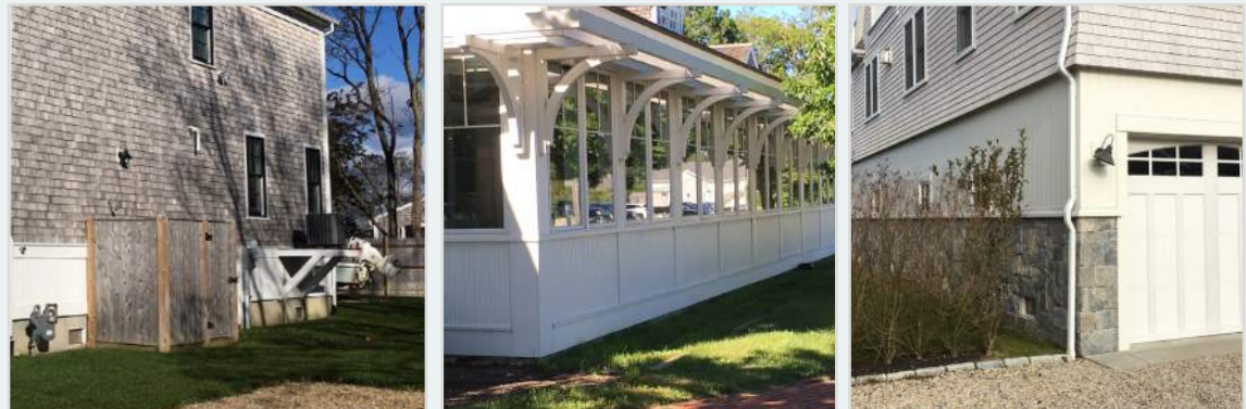
Building retrofits include elevating mechanical systems (left), filling basement areas, dry floodproofing (center), wet floodproofing (right), and elevating the interior first floor.
