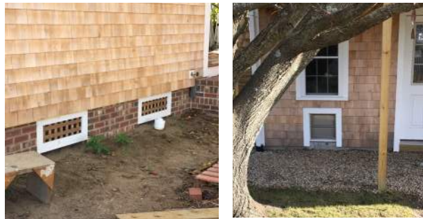
Flood vents allow water to flow in and out of unfinished and finished living spaces.
