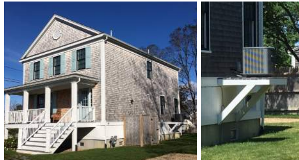
Raised platform on rear portion of side elevation for elevated mechanical equipment.
