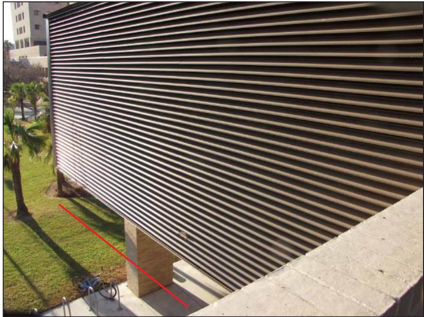
Figure 5-14. Example of protected emergency power system components. The BFE (shown approximately in red) is below the second floor so primary components of the electrical system were elevated well above the required flood elevation.
