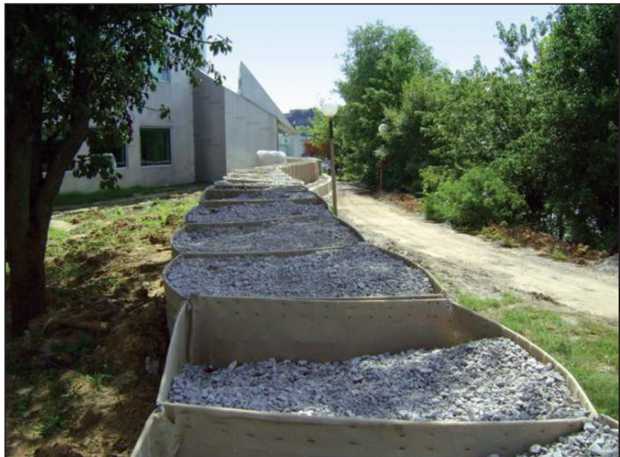
Figure 3-6. Gravel-filled containers formed a barrier to protect University of Iowa facilities during a flood event (2008).
