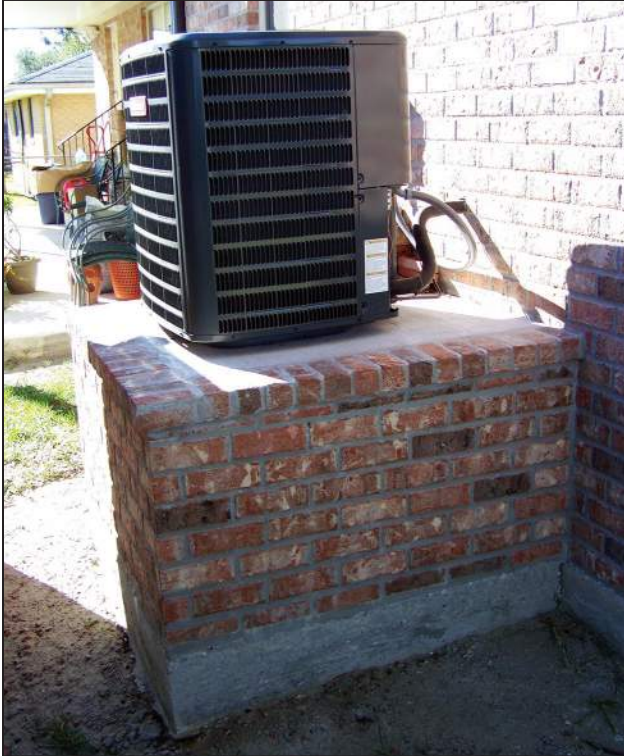
Figure 3-1. Air conditioning compressor elevated on a pedestal.
