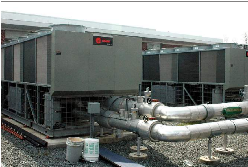
Figure 5-3. Air-Cooled rooftop chiller in Georgetown, Delaware.
